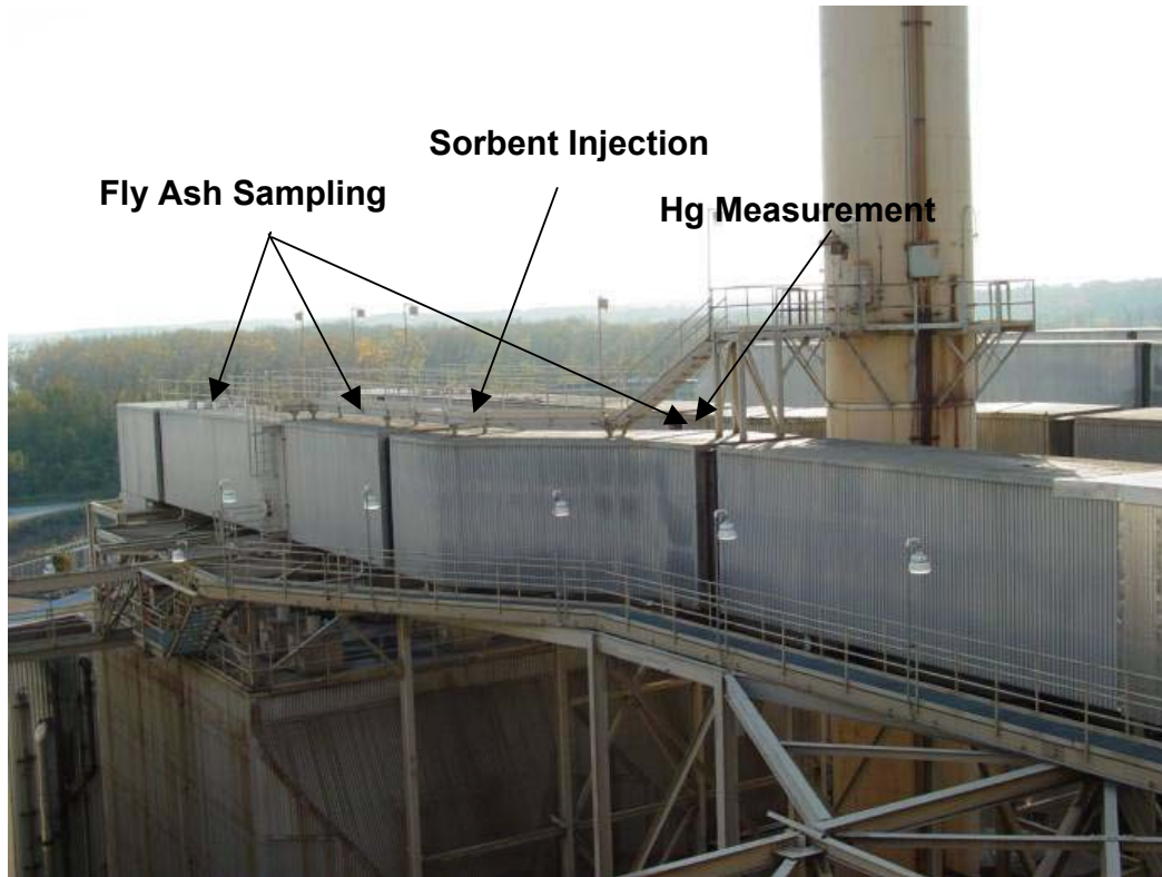
Figure 3. Photo of East ESP Inlet Duct, Meramec Unit 2.
