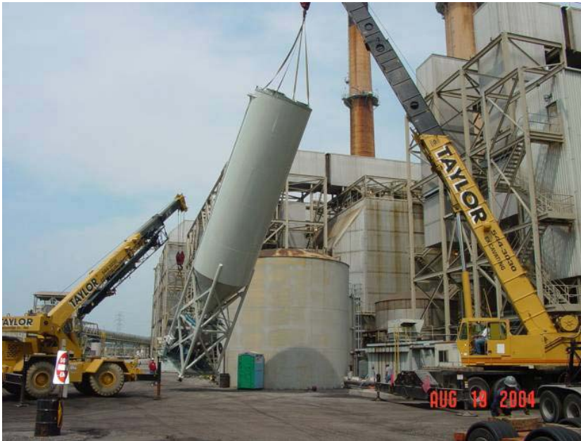
Figure 4. Photo of Injection Silo Installation at Meramec.
